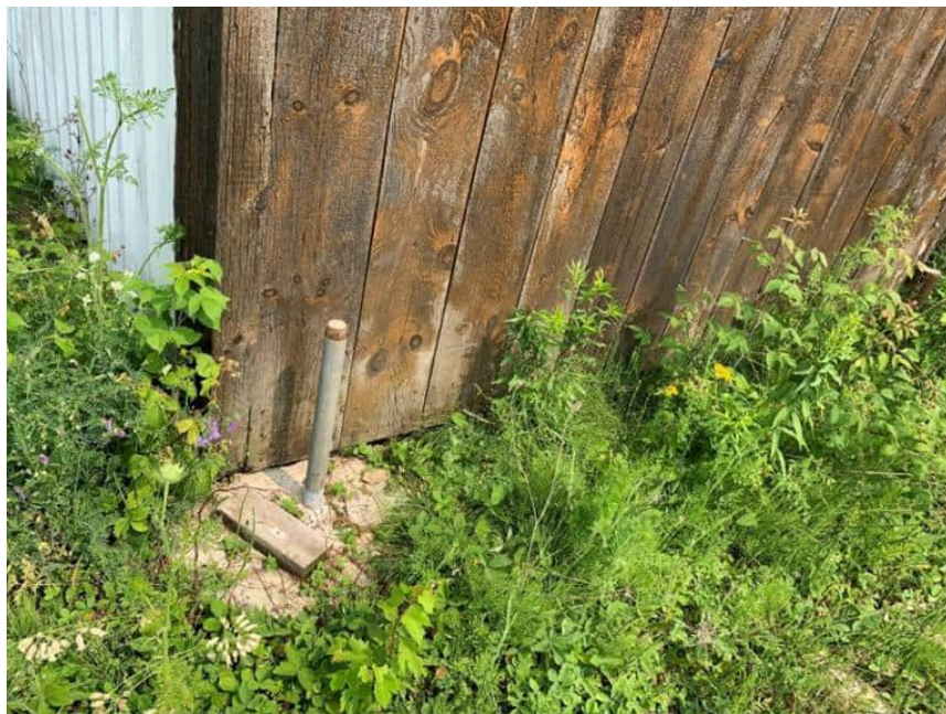
Photo 10: A view of the bottom of the structure in the western portion of the study area (potential snake hibernacula), June 29, 2023.
