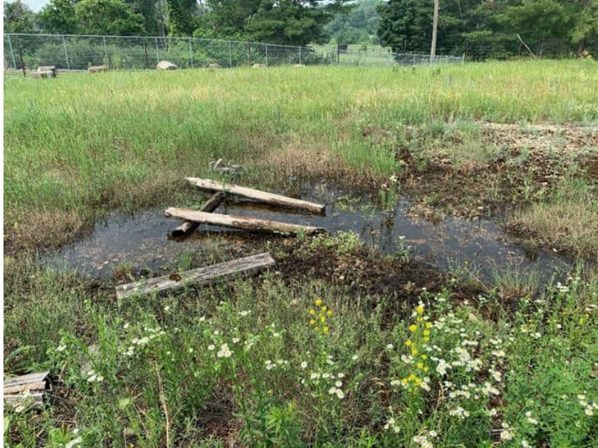
Photo 9: Existing conditions, illustrating poor drainage within the northwestern portion of the property, June 29, 2023.
