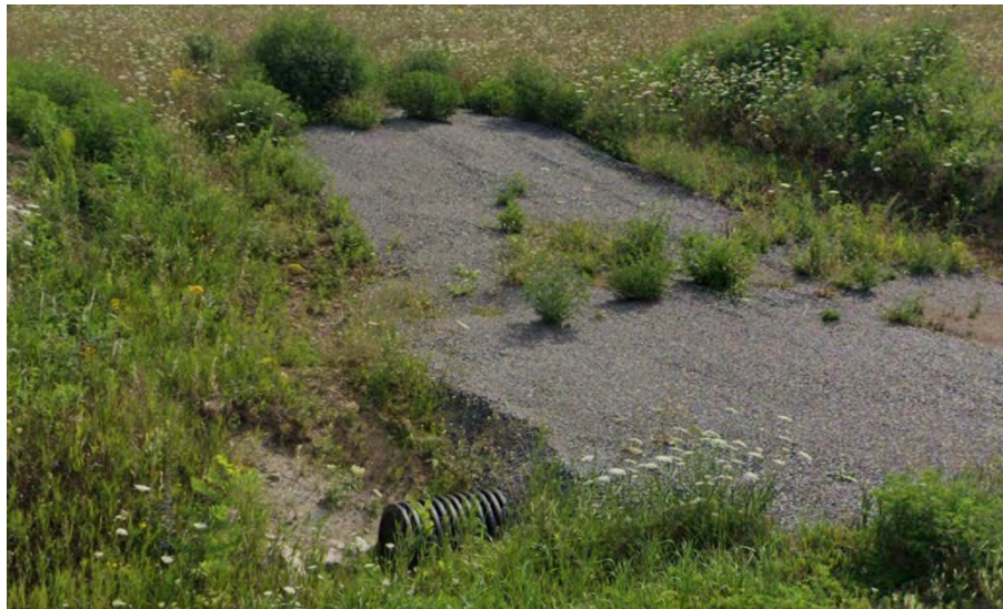
Image 11: One of two old driveways built over drainage ditch along Rosedale Road, view east.
