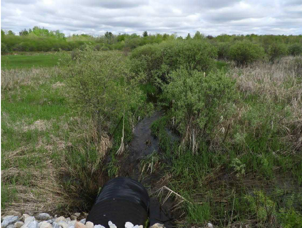
Photo 35: Culvert inlet on North Street conveying a tributary of Tay River within the Cattail Graminoid Organic Meadow Marsh (MAMO1-2) vegetation community in the southeast end of the study area. 24 May 2019.
