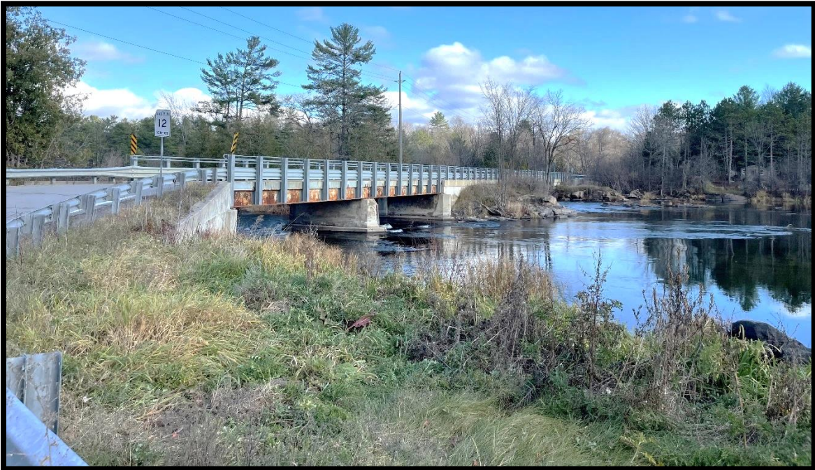
Figure 9: View of the upstream (south) side of the Blakeney Bridge looking from the west side. Source: Contentworks, November 2022.
