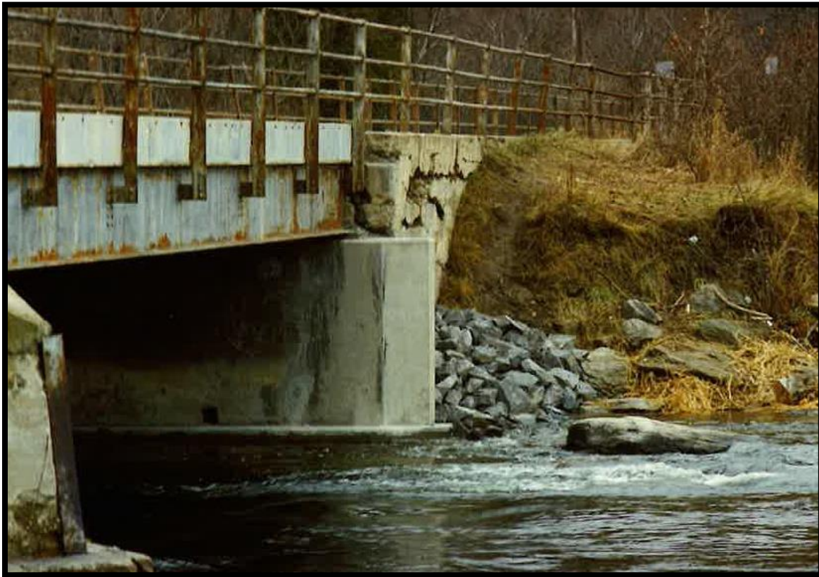
Figure 23: Photograph of the abutment requiring repair, 1993. The original railing, composed of riveted steel posts and steel piping is visible in this photograph. The railing system was replaced in 2000 with the current guardrails with handrails. Source: County of Lanark, Repair Photos 1992, Blakeney Bridge
