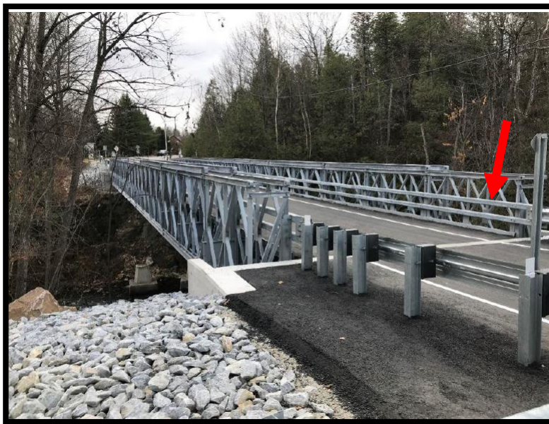
Figure 66: Bolingbroke Bridge, Tay Valley, completed in 2021. The bridge will have a very similar appearance to this bridge, but with three rails instead of two on the railings (arrow). Source: Lanark County, “Blakeney Bridge Report #PW-26-2022,” prepared for the Lanark County Public Works Committee, 26 October 2022.
