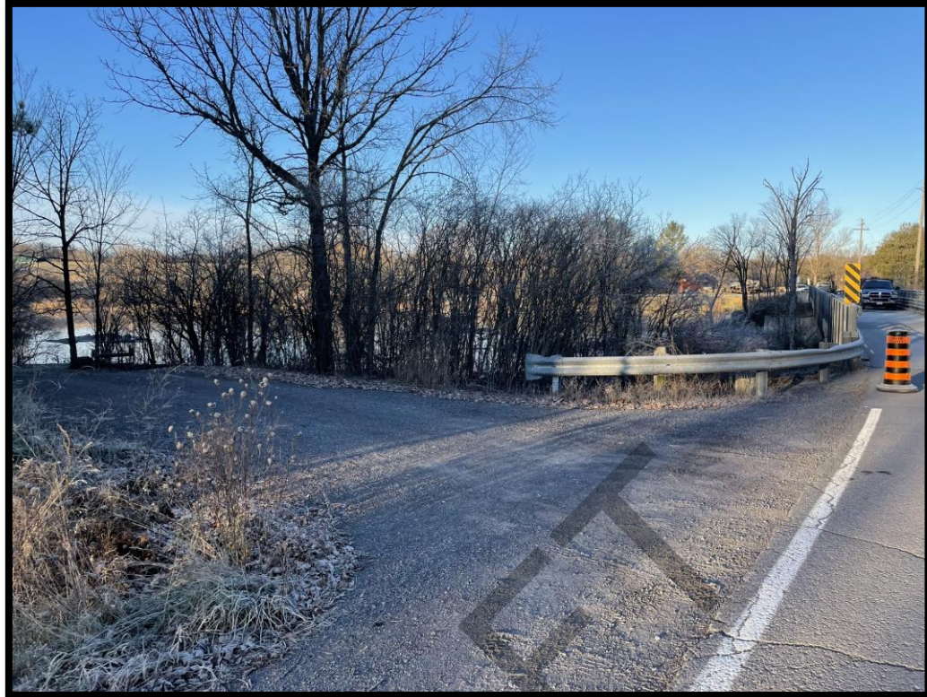
Figure 15: Gravel driveway disturbance beside bridge. (MH1149-D005)
