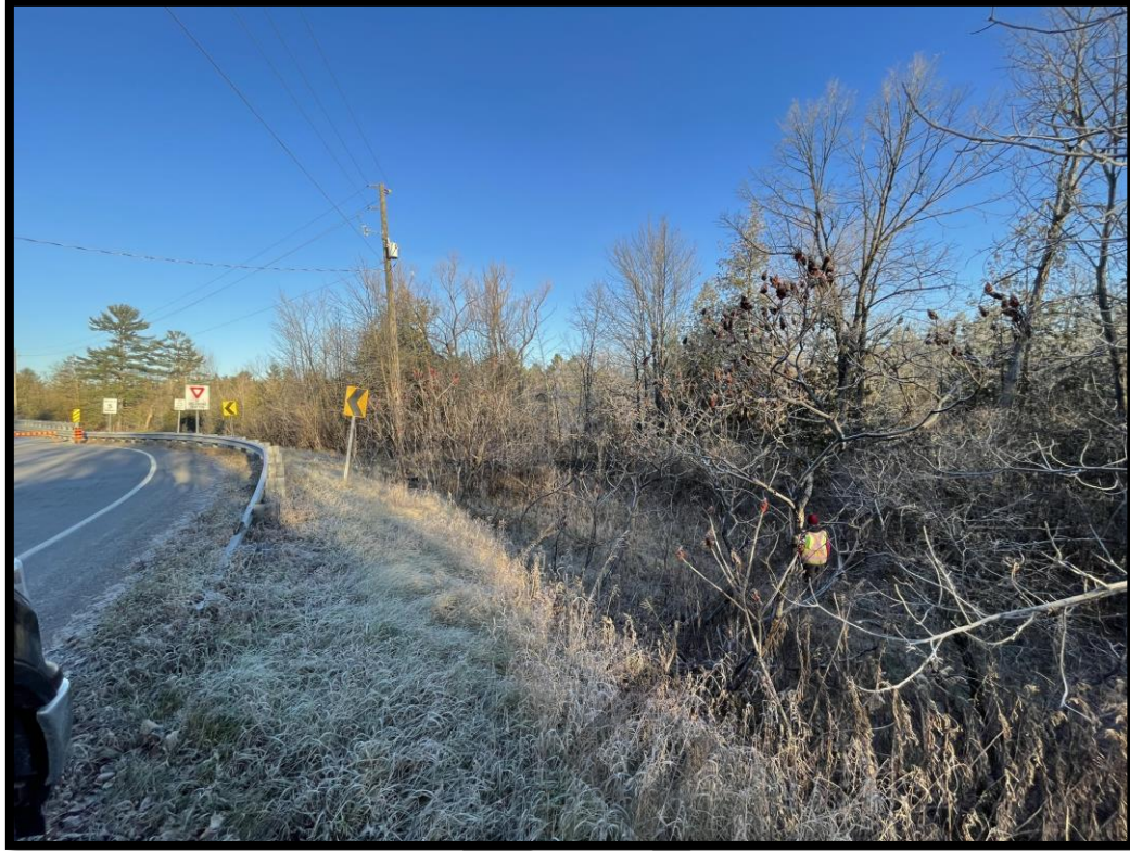
Figure 13: Steep embankment on the approach to the bridge on the eastern side leading to study area. (MH1149-D002)
