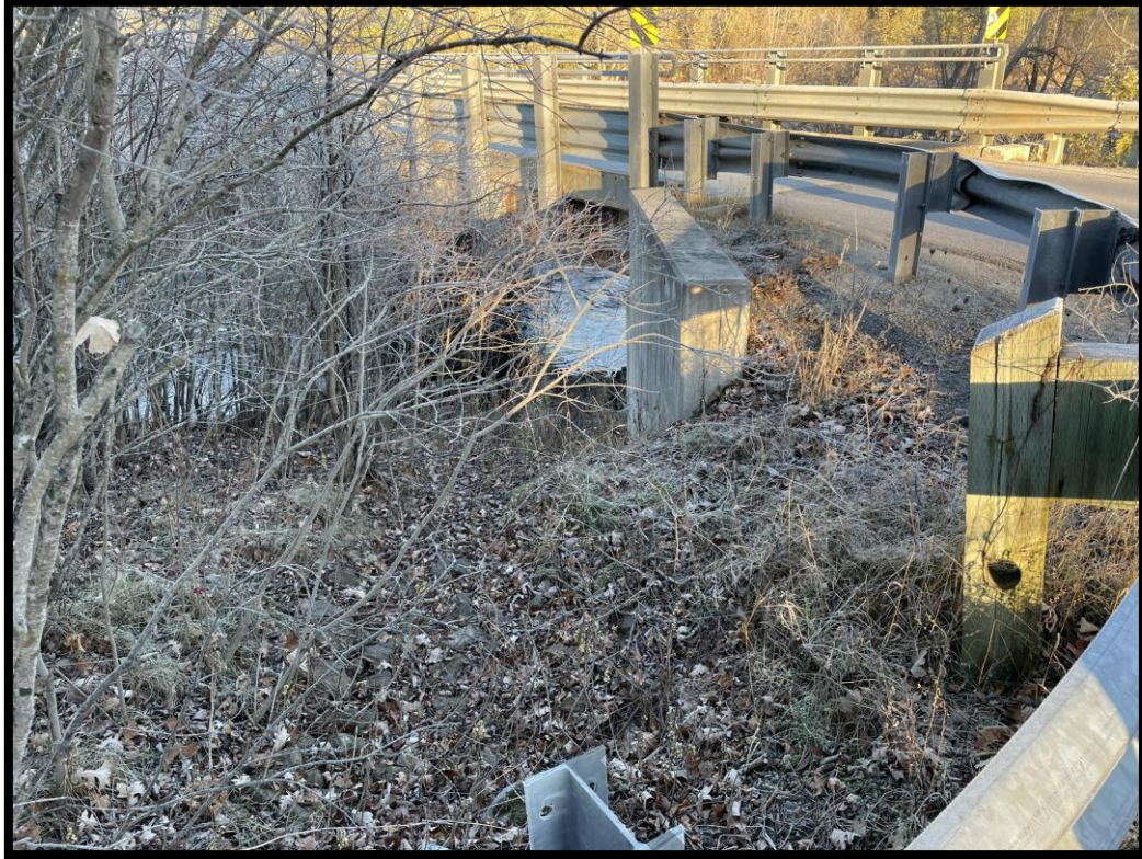
Figure 5: Bridge supports and previous disturbances. (MH1149-D006)
