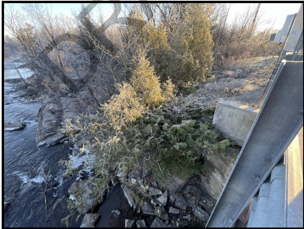
Figure 12: Steep bedrock outcrop with no soils in the middle of the river that the bridge is built on. (MH1149-D007)
