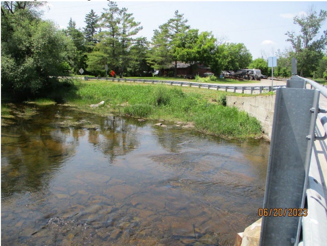
Photo 8 – Looking westerly at the SW corner of the current bridge. It is in this area that most of the changes to the bridge alignment will occur.
