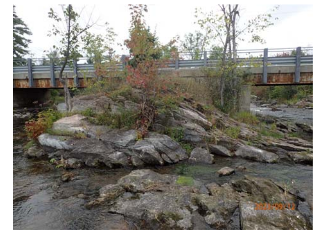
SOUTH RETAINING WALL BETWEEN EAST ABUTMENT MIDDLE BRIDGE & WEST ABUTMENT EAST BRIDGE
