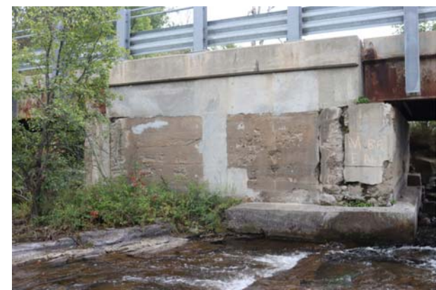
NORTH RETAINING WALL BETWEEN EAST ABUTMENT MIDDLE BRIDGE & WEST ABUTMENT EAST BRIDGE
