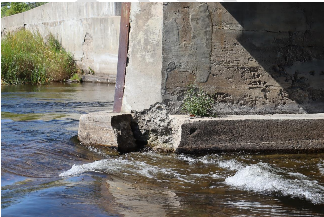
Image 46. Fractured pier collar of west bridge pier east side
