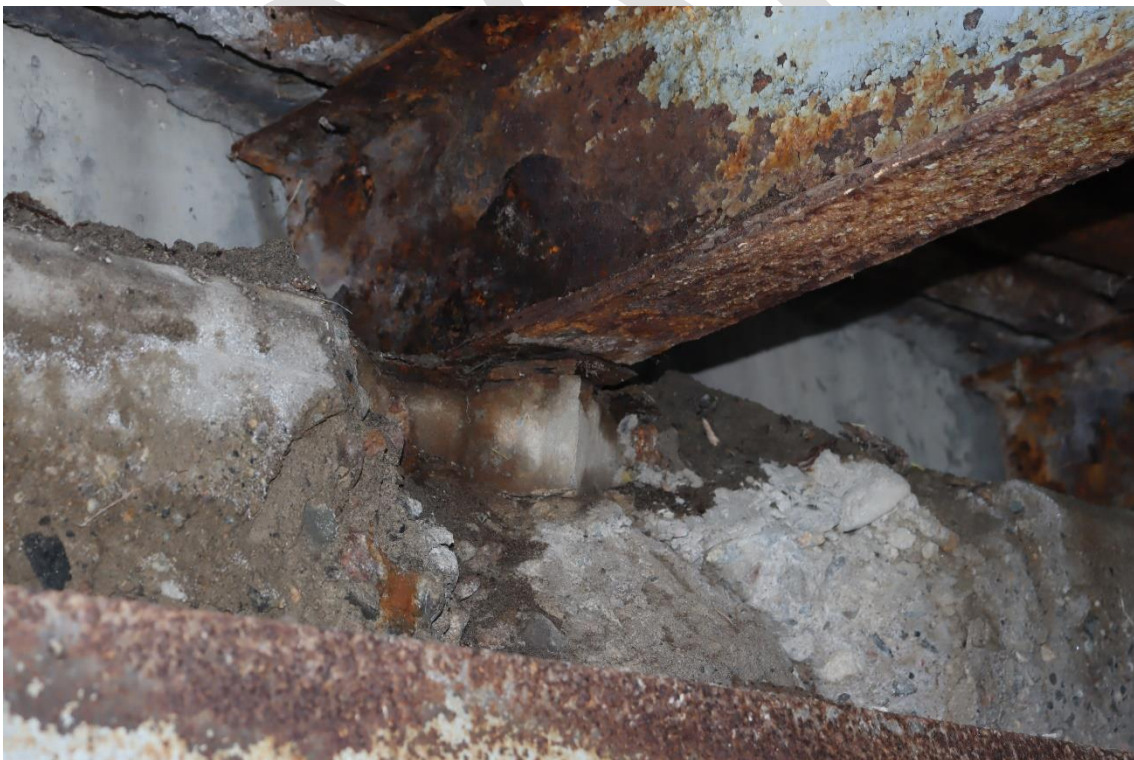
Image 27. Disintegration of west bearing seat of west bridge at Stringer 3
