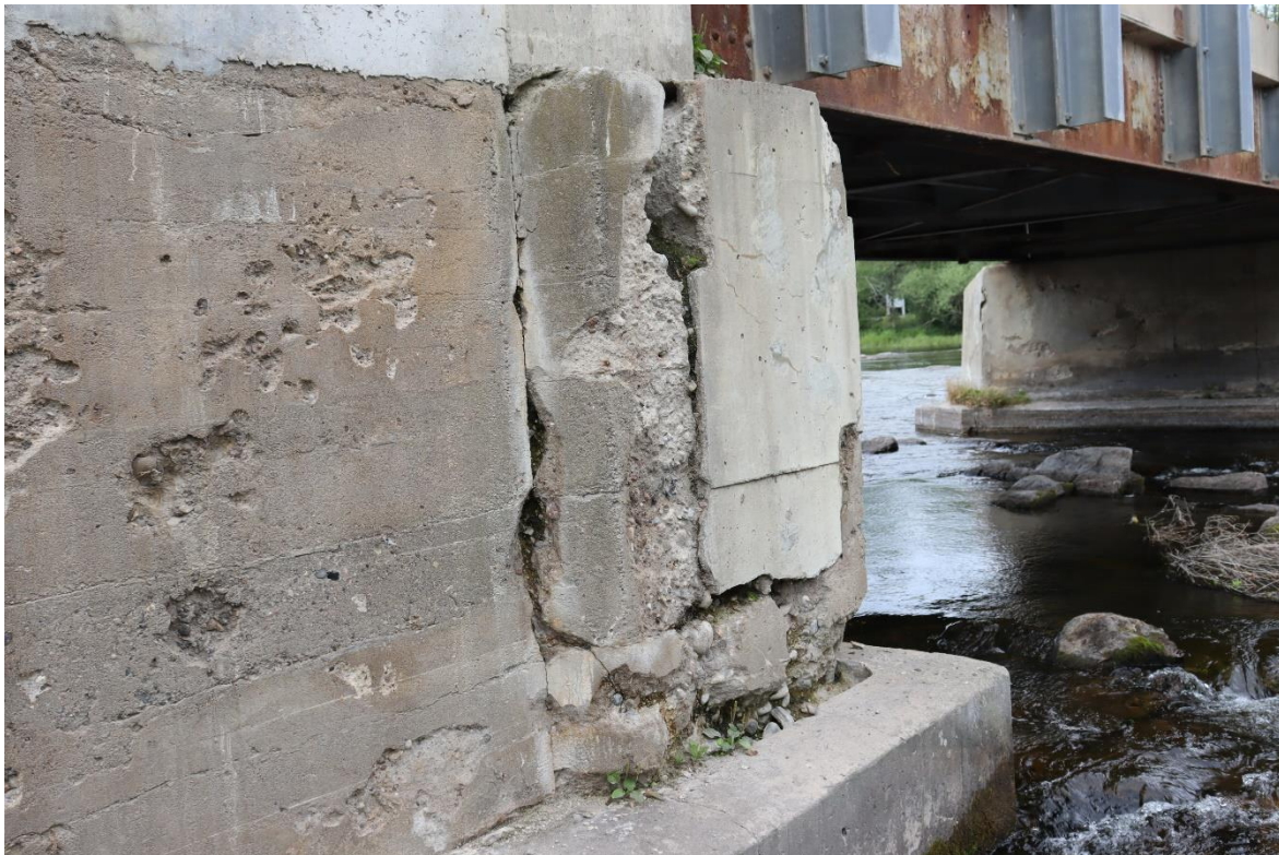
Image 4 Severely deteriorated substructure concrete with prominent patch
