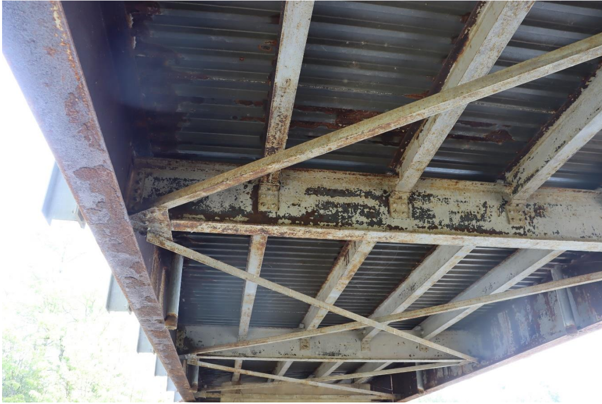
Image 7 Typical steel floor system with exterior main girders, transverse floor beams, and longitudinal internal stringers
