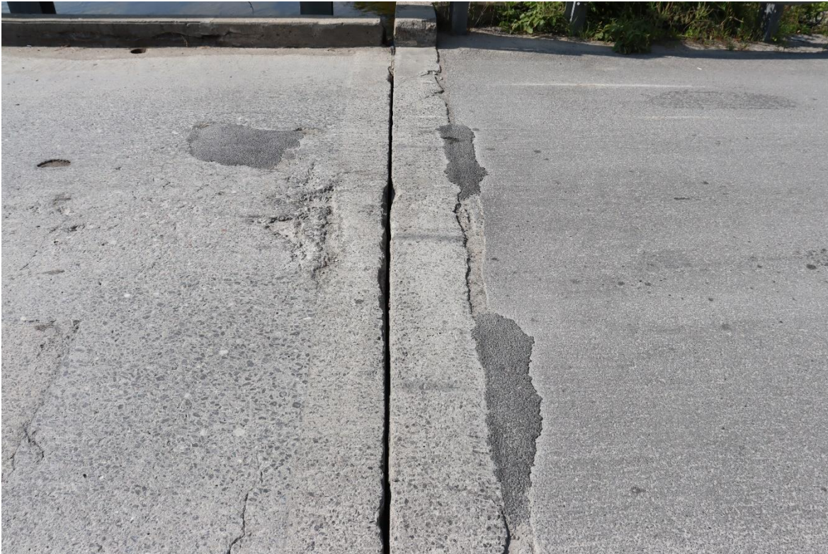
Image 6 Typical deck end and open expansion joint that admits chlorides to girder ends
