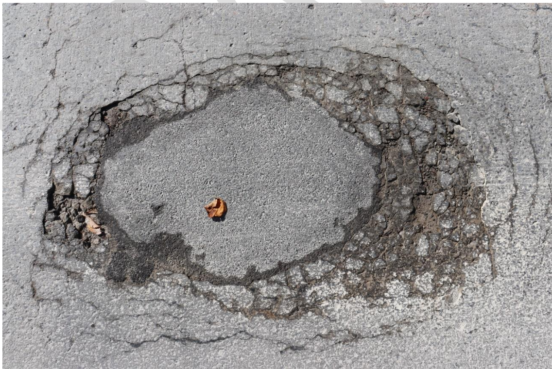
Image 5. Concerning pothole cracks with asphalt patch on deck of middle bridge
