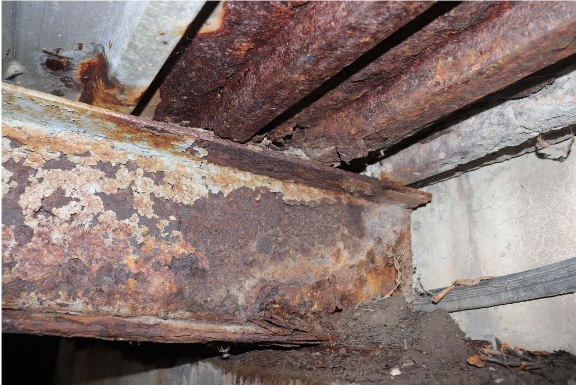
Image 15. Perforation of 3rd stringer from south of middle bridge west abutment
