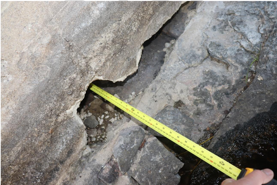
Image 14. West abutment 1.2 m deep cavitation undercut, east bridge
