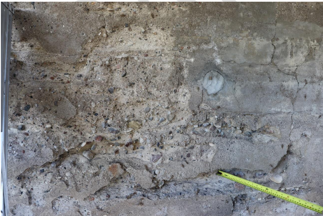
Image 8. East abutment disintegration and spalling of east bridge to 100 mm depth
