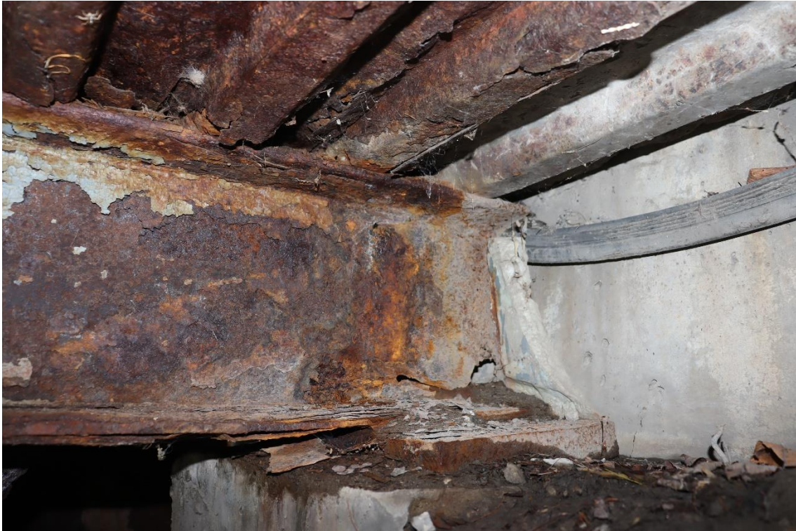
Image 13. Perforation of 1st stringer from south of middle bridge west abutment
