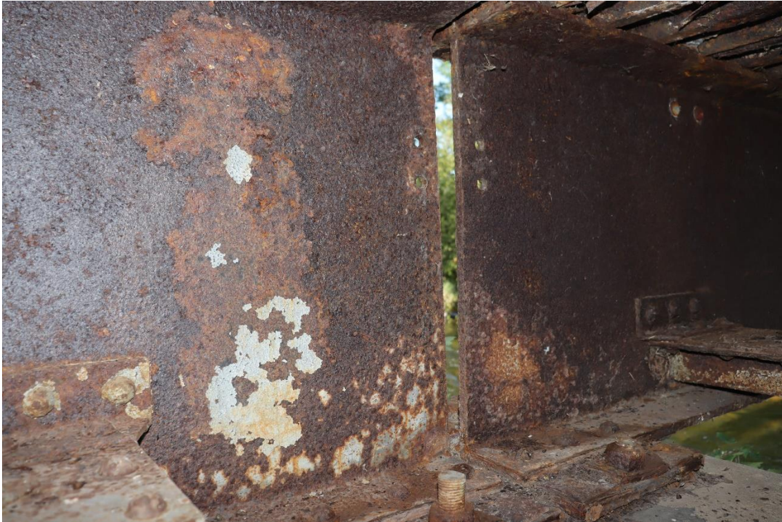
Image 47. Condition of girder ends on pier of west bridge
