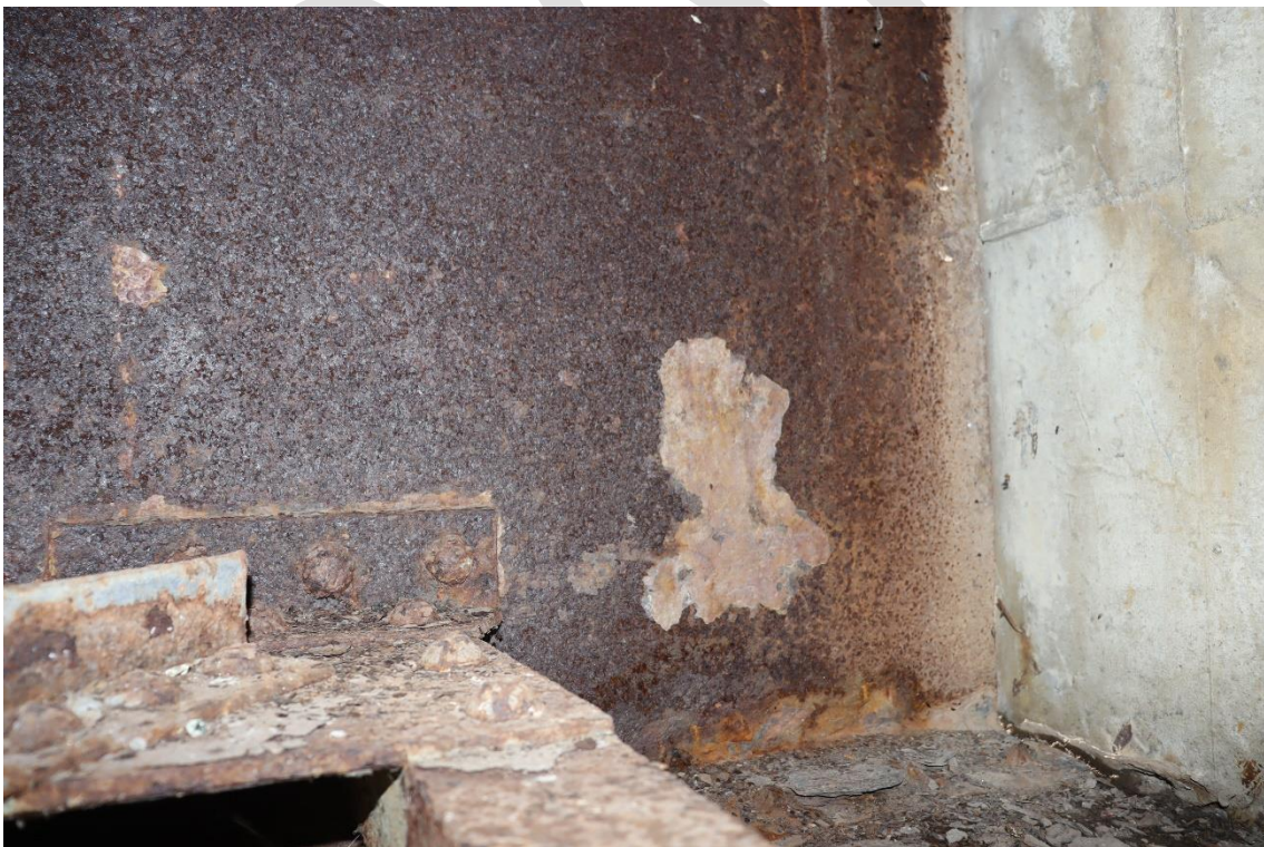
Image 30. Web thinning of south girder end of middle bridge west abutment
