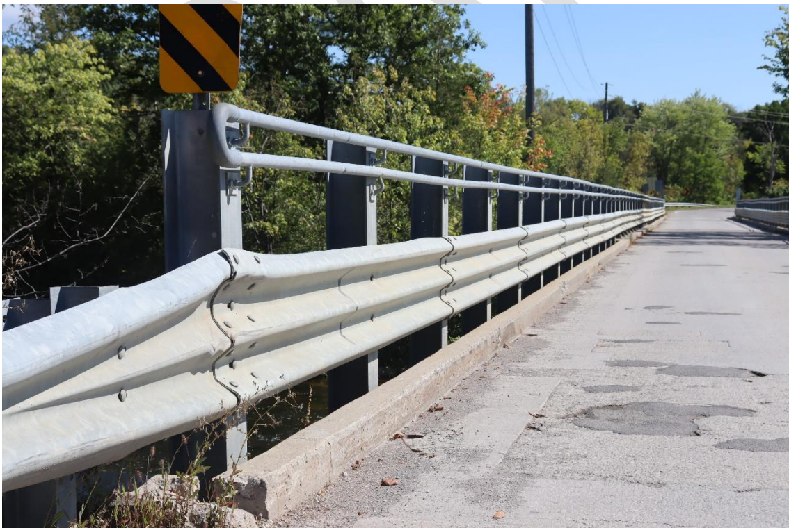
Image 38. Typ. guide rail on west bridge and asphalt condition
