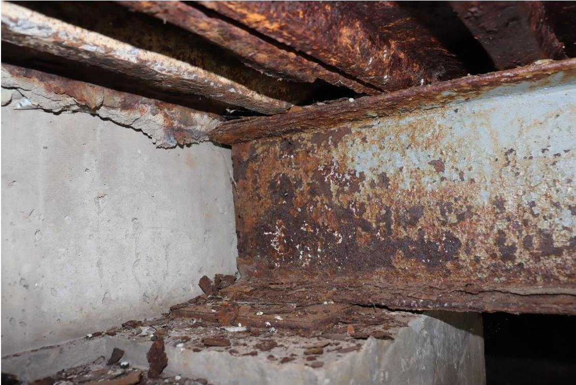
Image 4. Typ. condition of stringer west end of east bridge
