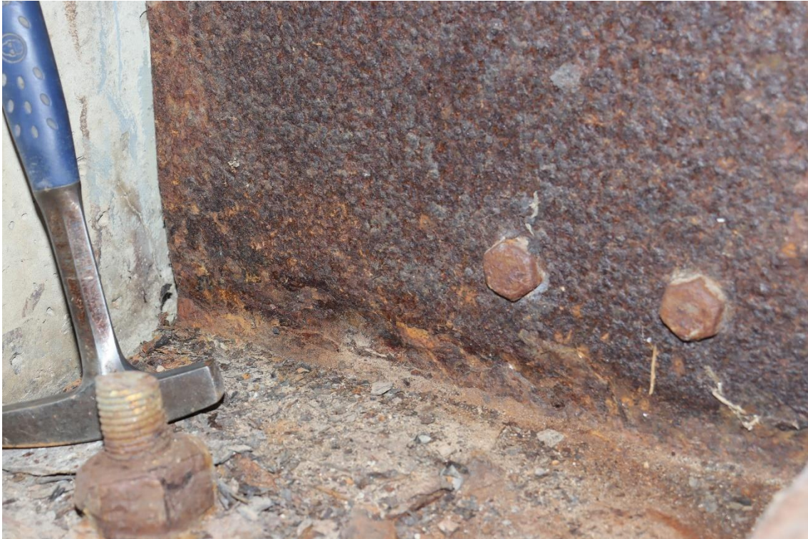
Image 11. Web thinning of south girder east end of east bridge
