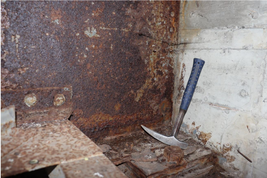
Image 43. Web thinning of north girder end on east abutment of west bridge
