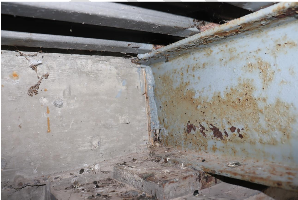
Image 22. Typ. condition of stringer east end of west bridge
