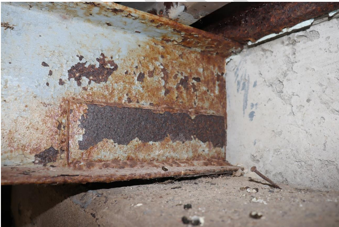
Image 12. Web patch on 3rd stringer from south on east abutment of east bridge
