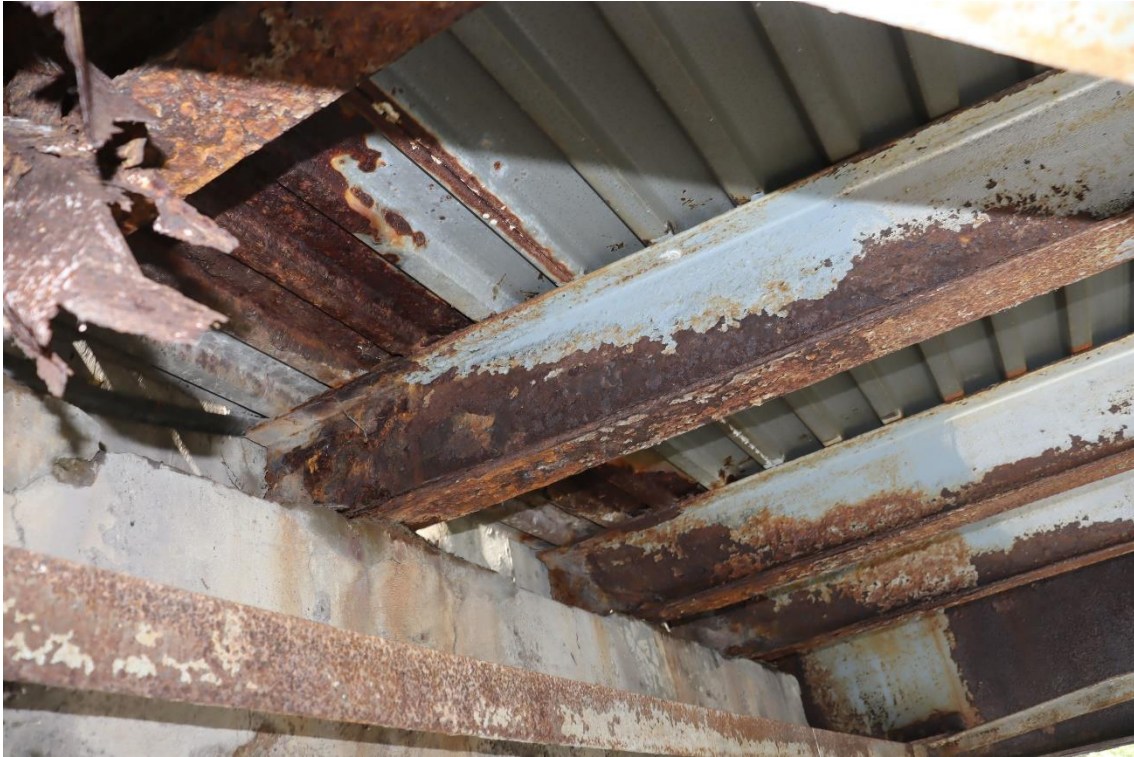
Image 29. General condition of stringer ends of middle bridge at west abutment
