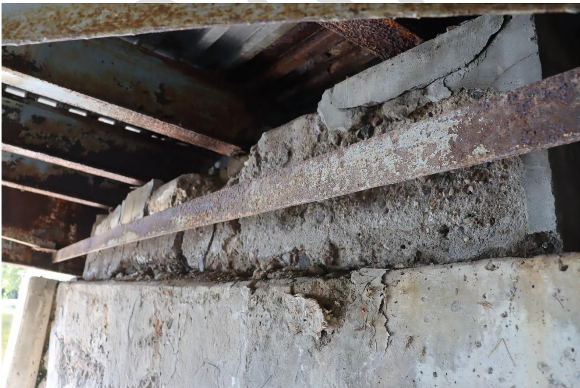
Image 25. Disintegration of ballast wall above west abutment of west bridge
