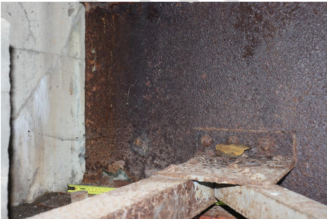
Image 52. Perforation of north girder end on west abutment of west bridge
