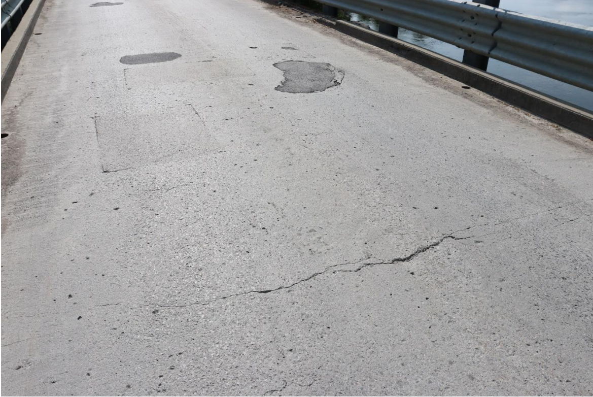
Image 5 Typical deck with concrete patches, cold patches, cracking, and delamination
