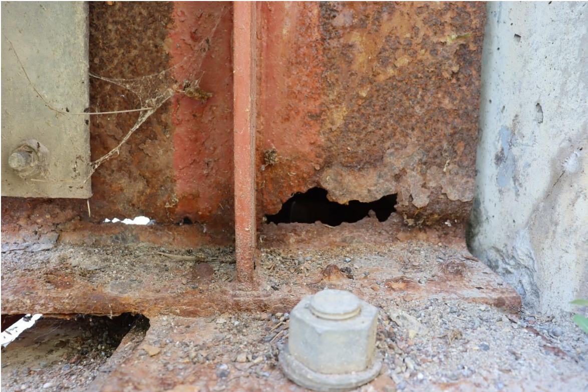
Image 2 Perforated main girder north side of west span at west abutment, with strengthening added
