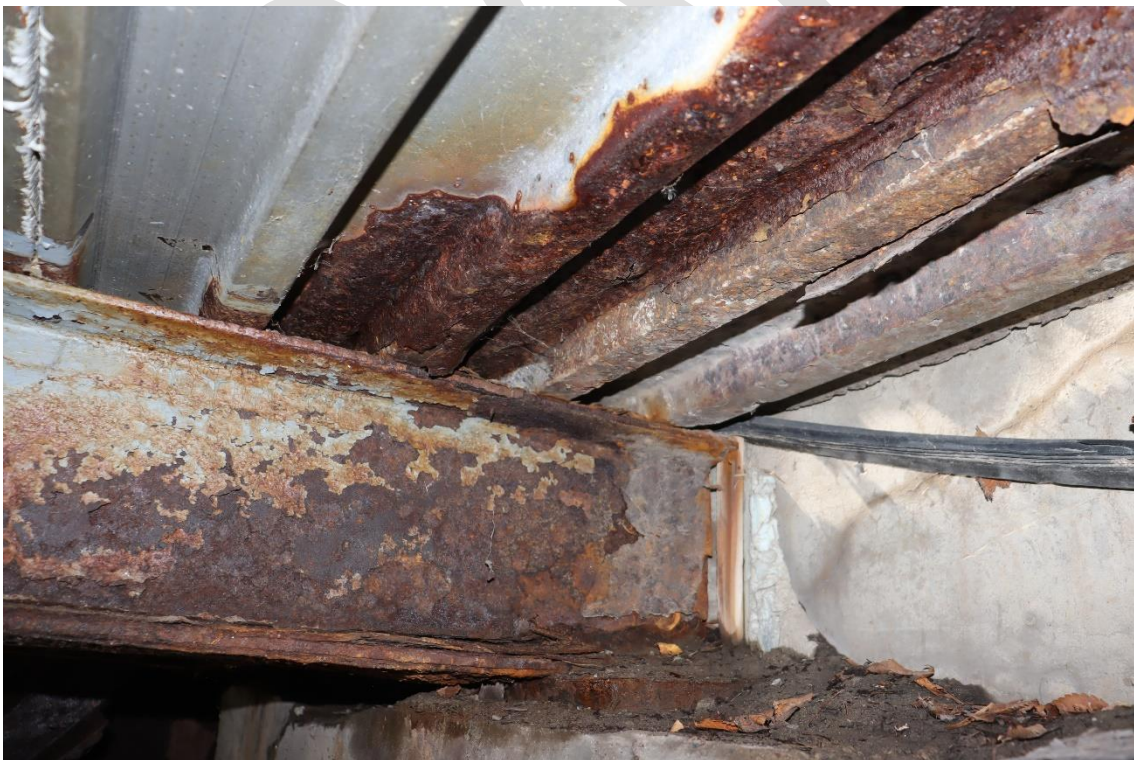
Image 14. Perforation of 2nd stringer from south of middle bridge west abutment
