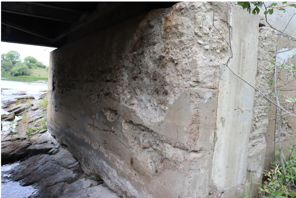
Image 8 Severe disintegration of 1912 concrete and undercutting of foundation at bedrock surface
