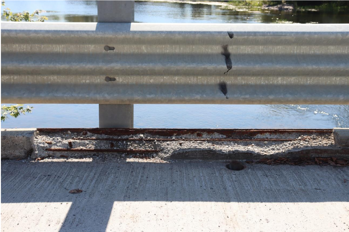
Image 39. Disintegration of south curb of west bridge
