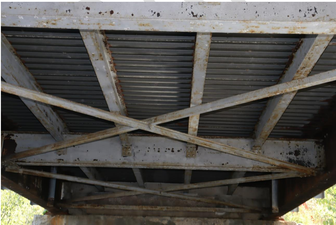
Image 9. Soffit & steel floor system of east span of middle bridge facing east
