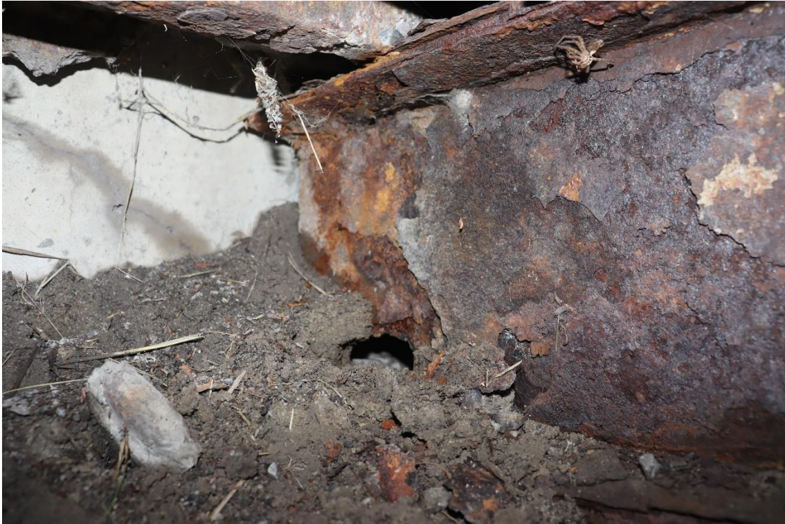
Image 26. West end of Stringer 2 with debris and perforation on west bridge
