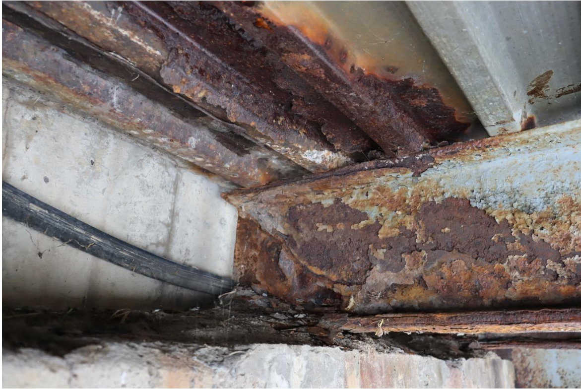
Image 3 Severely corroded stringer end on middle bridge, west end
