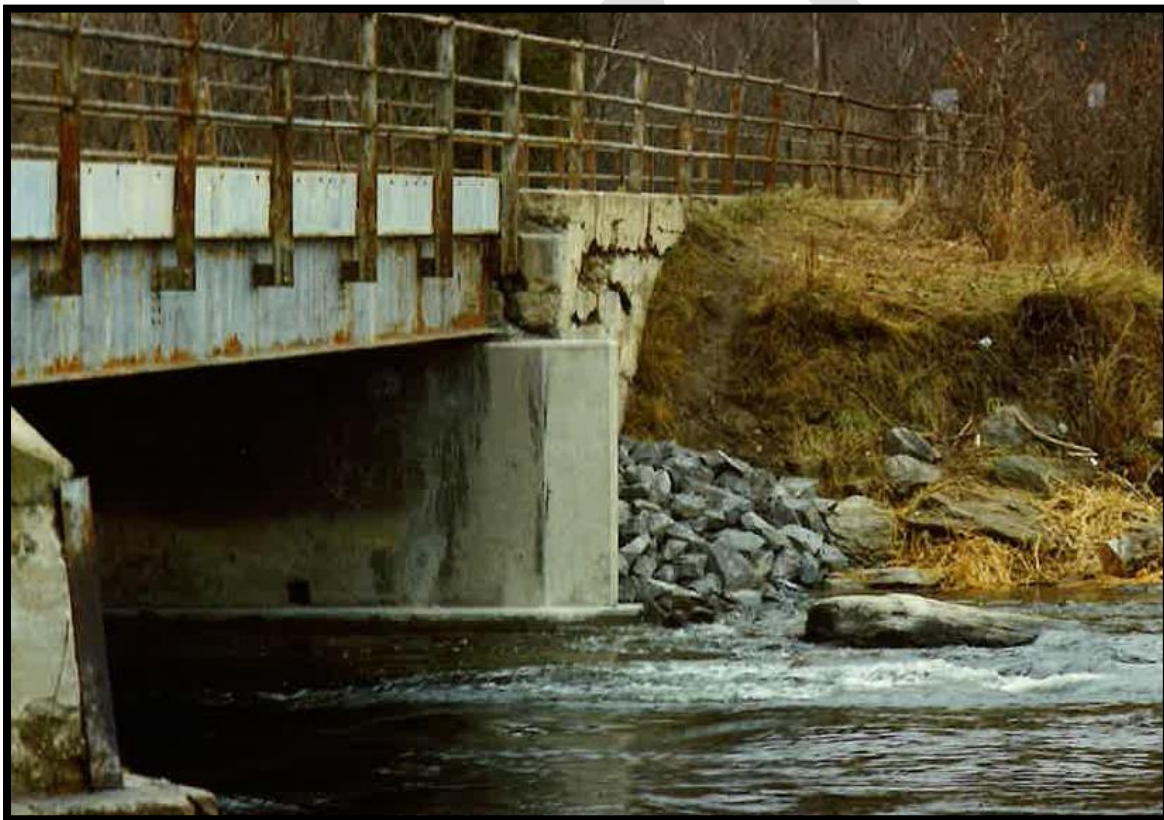
Figure 23: Photograph of the abutment requiring repair, 1993. The original railing, composed of riveted steel posts and steel piping is visible in this photograph. The railing system was replaced in 2000 with the current guardrails with handrails. Source: County of Lanark, Repair Photos 1992, Blakeney Bridge
